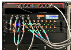
Name : CH-Grid-4Port-5 IP Address : 192.168.0.139 Details : 4 DMX output 2 Isolator(1 to 8 / 2 to 4) A1~A4 is for Chauvet Ovation
